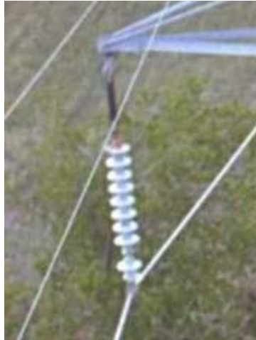
Fig. 2. Broken insulator unit (developed at Electric Power Research Institute).
